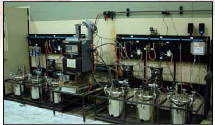
New paint mixers ensure the most efficient mixing and storage for vehicle and equipment paint. This not only reduces the likelihood of spills, but also simplifies operations for CSMS painters. Paint mixers also reduce waste by keeping paint fresh, avoiding the disposal of unused paint.
